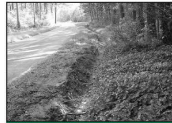
Bare soil in this ditch will erode and contribute to pollution downstream. Photo by Bruce Nichols, NRCS
