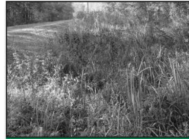
A wide, shallow drainage area can reduce erosion and control sediments. Photo by Bruce Nichols, NRCS
